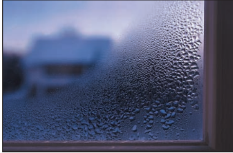
Condensation on the inside of a window-pane.
